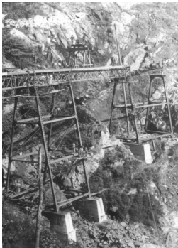
Construction of railway bridge across Stony Creek on the Cairns-Kuranda railway line (c.1890)
